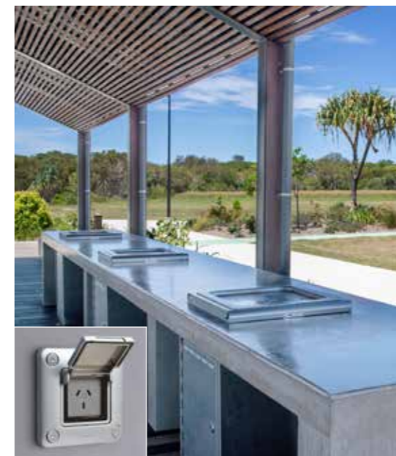
OUTDOOR AREAS | Weatherproof Powerpoints
