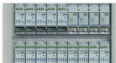
Area accessible to the installer with all the power supplies, actuators and other DIN devices (up to 288 modules) for the operation of the MyHOME system. The installation is completed with the white finishing panels.
