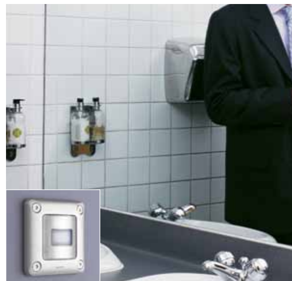
PUBLIC WASHROOMS | Automatic switch
